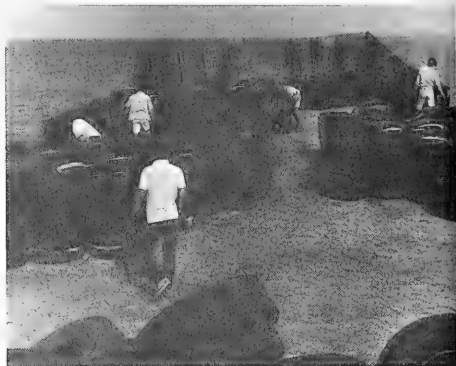
Figure 14.--Barge loading 7-tire units. The units have concrete ballast and are held together with tie-rods.
